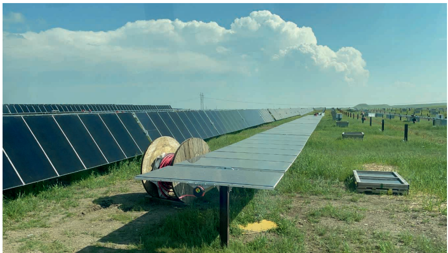
A look on the ground as crews prepare the Wild Springs Solar Project for power generation. Photo submitted by East River Electric
